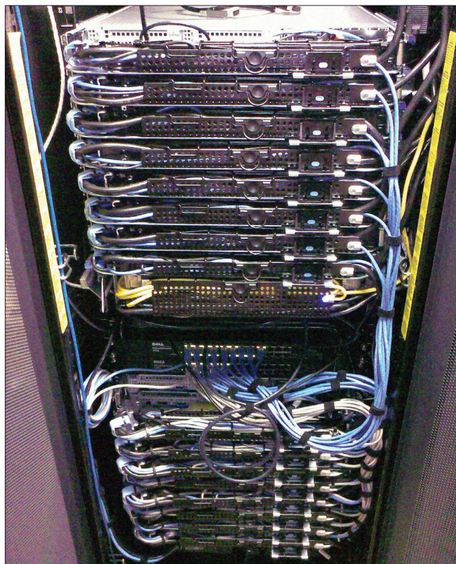
Figure 2: Cluster cabling can get out of hand quickly, so be neat.
