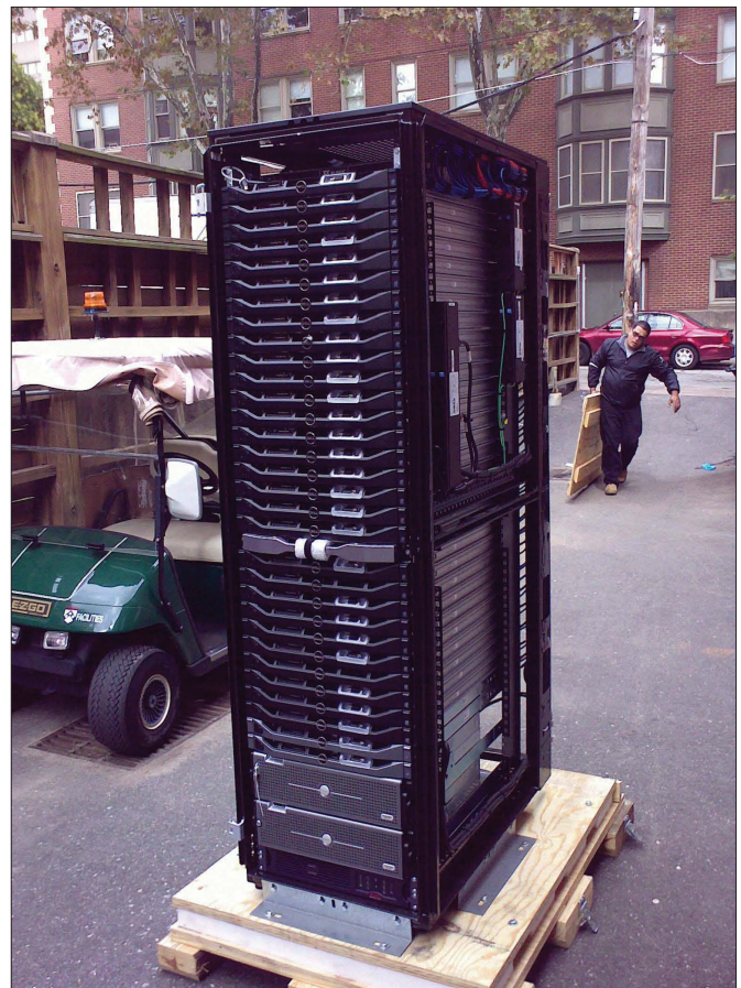
Figure 1: A new cluster still on the pallet.
